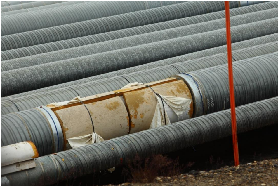
Exposed insulation that surrounds oil carrying pipes
