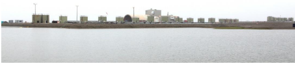
Row of oil wells capped with boxlike buildings surrounding a Christmas Tree
