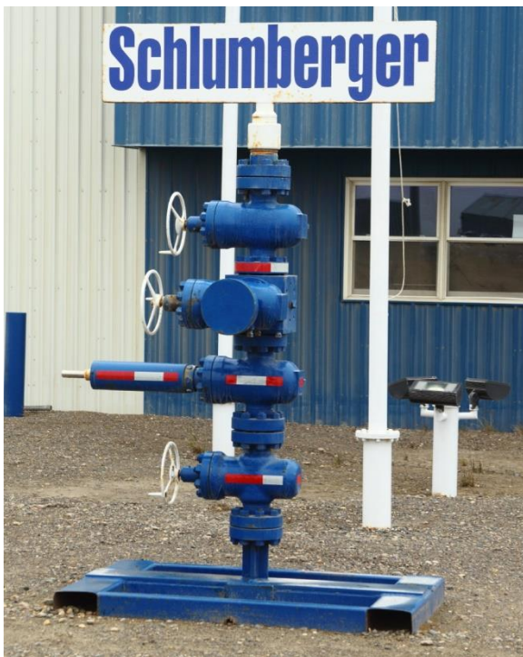
Example of a Christmas Tree capping each oil well
