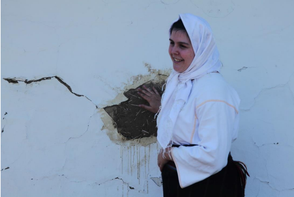
A needed repair
